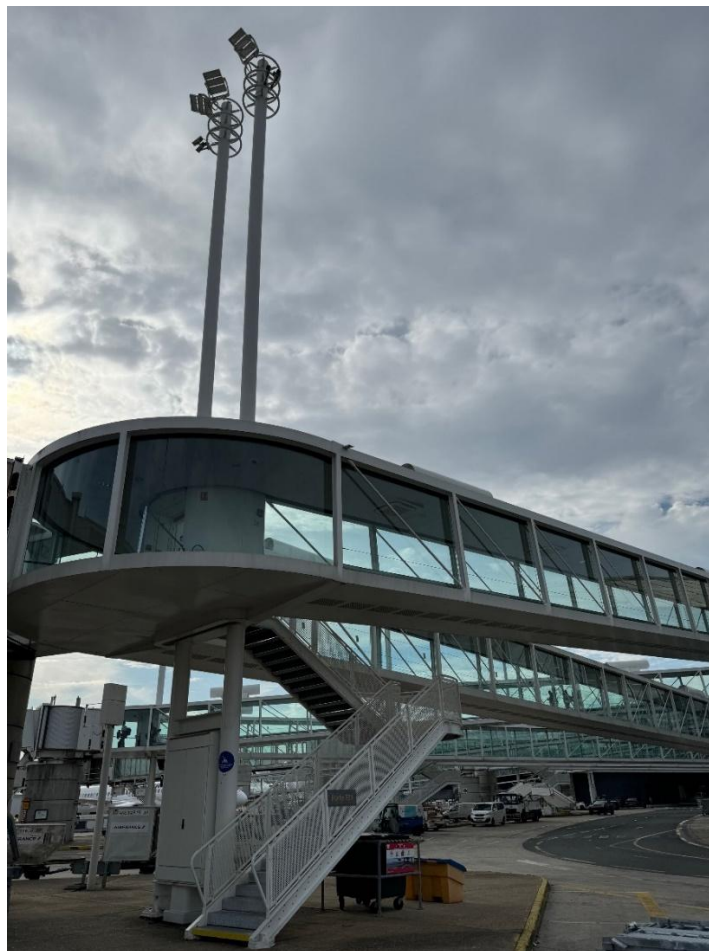
Figure 3: Terminal 2F poles with LED fixtures, and electrical cabinets
